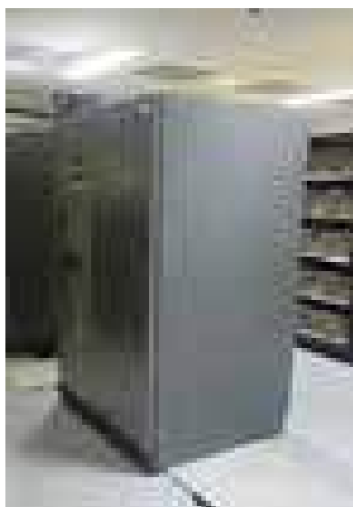
(Newly installed 200 kVA UPS)
